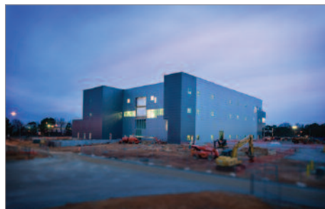
Grifols Fractionation Facility, Clayton, NC
